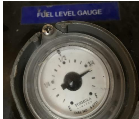
Standard gauge within the enclosure. These are okay, just inspect and make sure they are not cracked.
