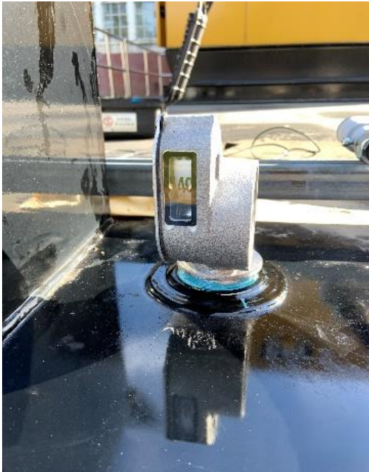
Morrison 718 Installed on outdoor tank
