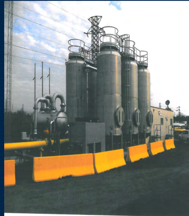
Hydrogen sulfide and siloxane removal vessels
