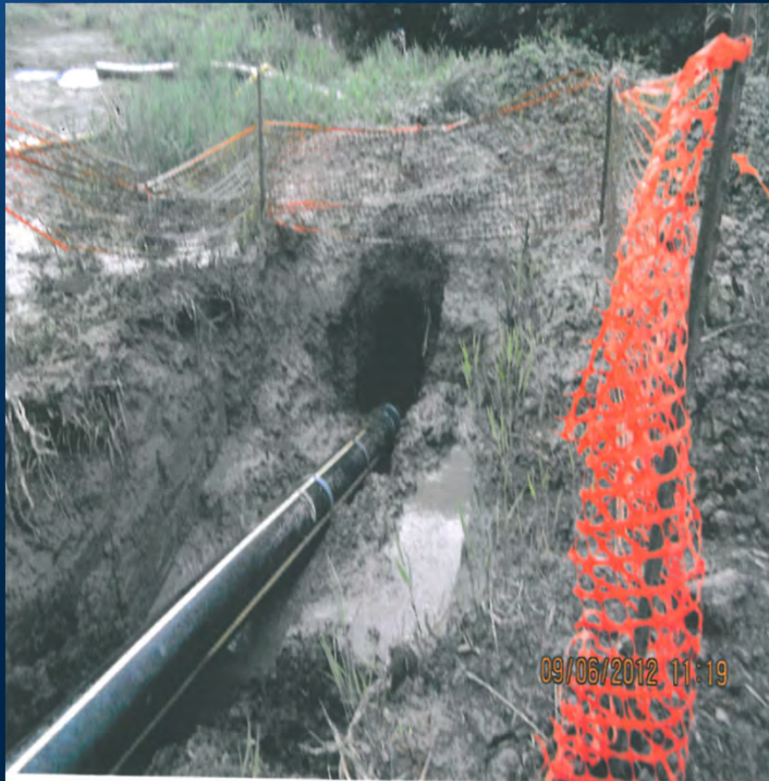
Open trenching, jack and bore and directional drilling methods were used to install transmission pipeline
