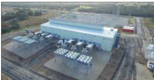
Sky Global provides power to an 8 county area using GE gas engines.
