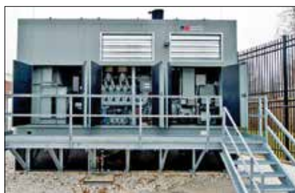
Outside the Cerner Technology Center, MTU Onsite Energy Series 4000 generator sets are contained in Level 2 sound attenuated enclosures.
