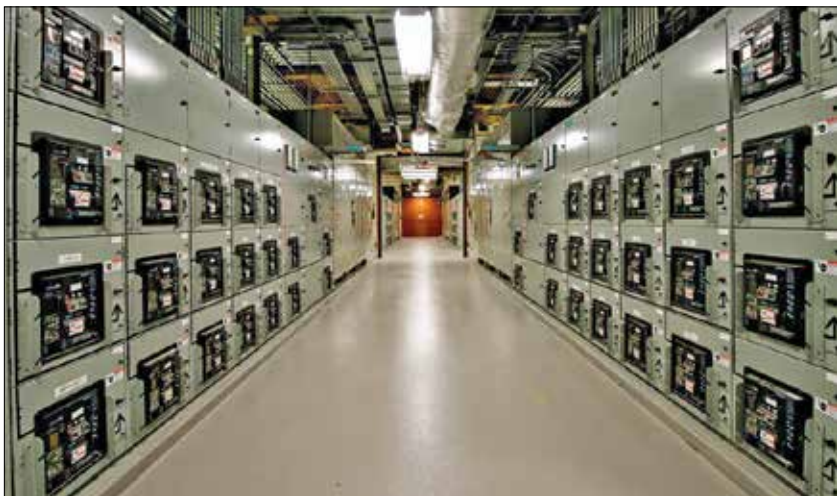
A sophisticated control system of Siemens PLCs coordinates the seamless operation of seven generator sets, four switchboards and two utility sources.
